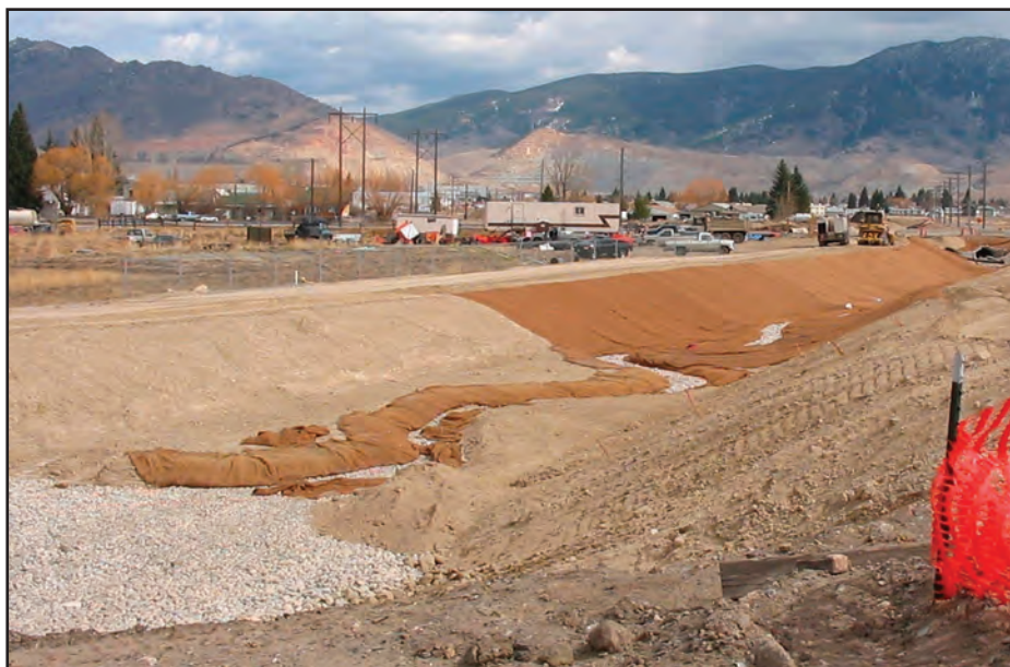
Final stages of channel reconstruction. One foot of gravel covers the entire channel bottom (lower left). The pilot channel and "floodplain" were created by placing one foot of soil over the gravel except in the meandering pilot channel (center). Soil was covered with erosion control fabric after seeding (right).
