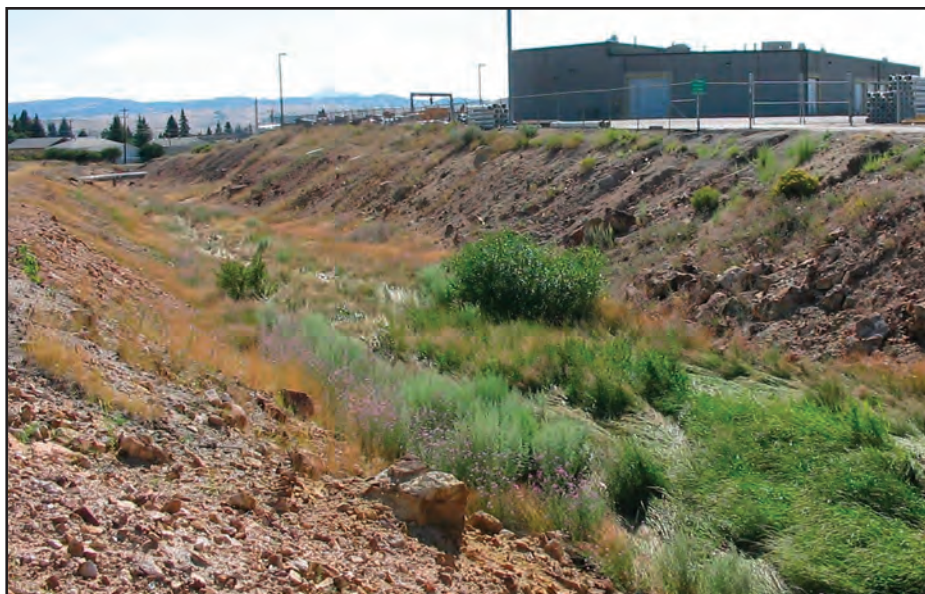
The Butte Metro Storm Drain before reconstruction and revegetation.
